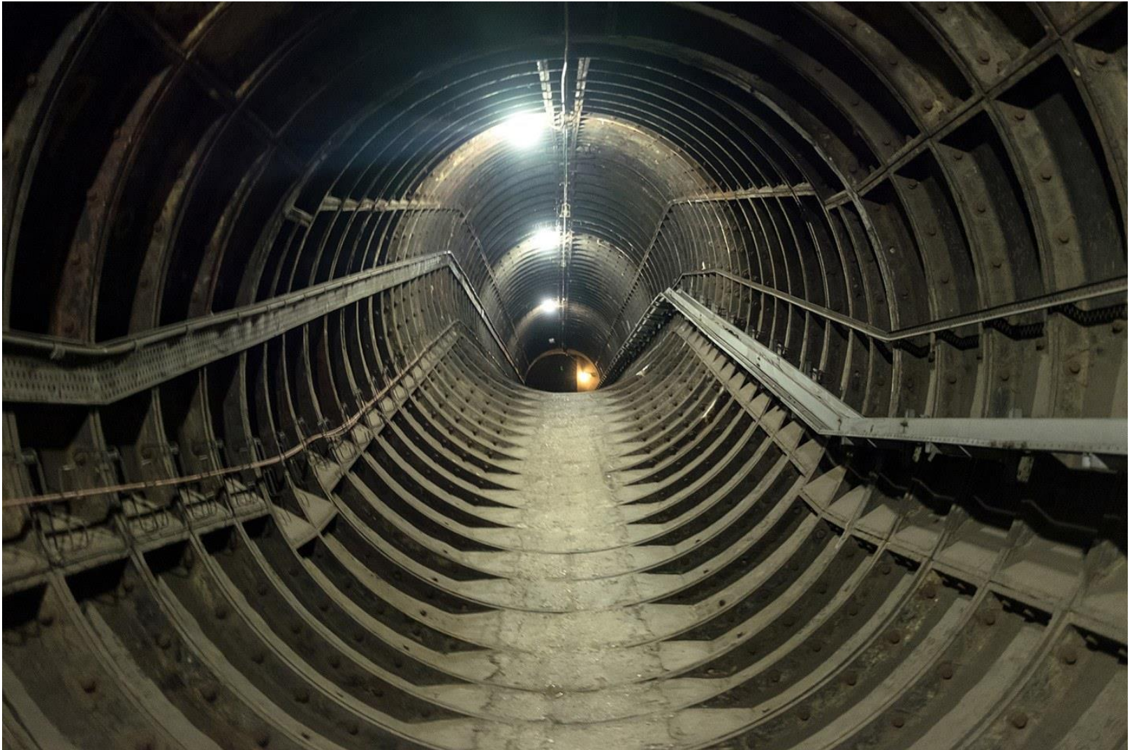
Part of the old tunnels at Euston this old Pedestrian tunnel is now used for ventilation on the Northern Line
